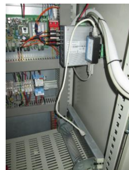
Cable Ethernet desconectado del switch/PLC Ethernet cable disconnected from the switch.
