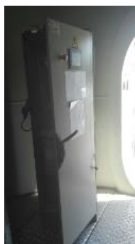
Armario Ground / Ground Cabinet
